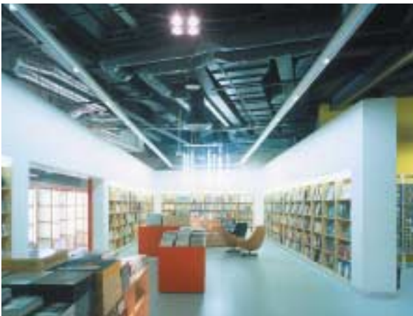
17. The bookshop, showing services integrated with structure.
